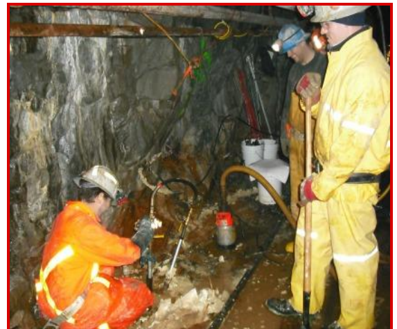
UNIVERSAL RESIN is used to stop water inflow problems for tunneling contractors.
