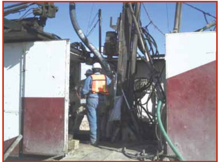
Excellon Resources, Platosa Mine, Mexico Deep hole drilling and high-volume cement grouting operations were used to seal water-bearing rock formations and successfully recover a flooded underground silver mine.
