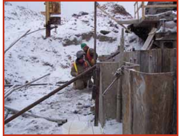
Agnico-Eagle, Goldex, Quebec Construction of a shaft collar through quick sand was overcome using a systematic engineered grout plan. The plan specified strategic placement of grout pipes as well as appropriate cement grout mixture for this unique application.
