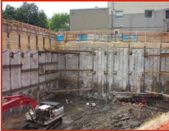
Deep Excavation, Cement Grouting, Toronto, Ontario Cement grout is routinely used to fill voids and seal water infiltrations in shored excavations.
