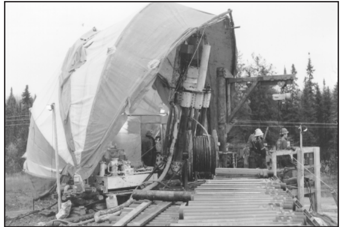
On this raise boring project, the 12-3/4" diameter pilot hole intersected underground water seams and was successfully tremie grouted from a depth of 330 m utilizing a motorized hose reel and swivel to place 21 m 3 of cement grout
