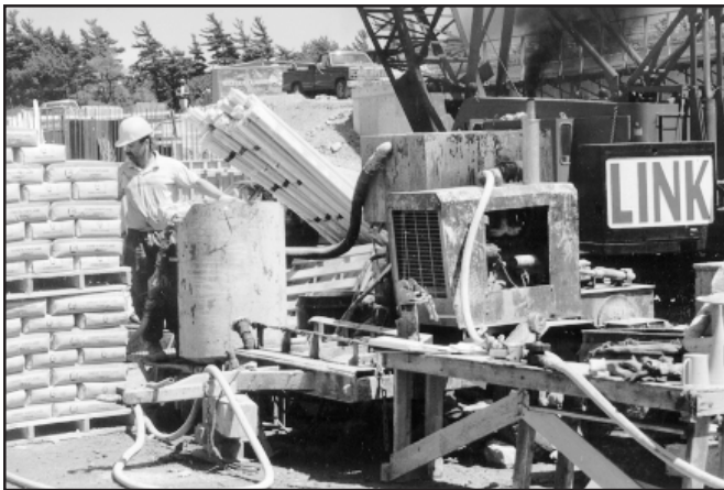
This highway bridge construction project utilized sleeve pipes, seen in the background behind colloidal mixer, for soil stabilization as part of the foundation design requirements
