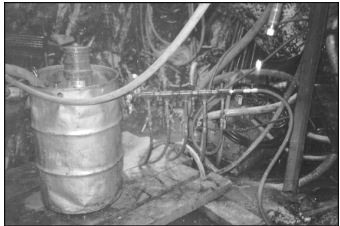
In a shaft sinking project that encountered fractured ground at a depth of over 200 m, microfine cement grout was pre-mixed and delivered to a grout pump located at the shaft bottom; a special grout manifold was fabricated that allowed up to six holes to be grouted concurrently until grout flow reached zero flow at maximum specified grouting pressure.
