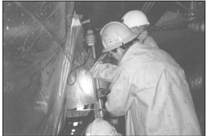
Grouting crew installing an inflatable packer prior to conducting water pressure test from within an inspection gallery located in the base of a large hydro power dam
