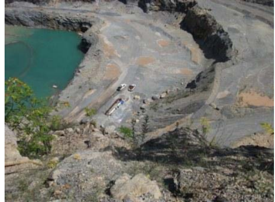
Pipes were set-up at the bottom of a quarry to test the effective delivery of the grout even when the equipment was located over 70 m higher than the point of injection
