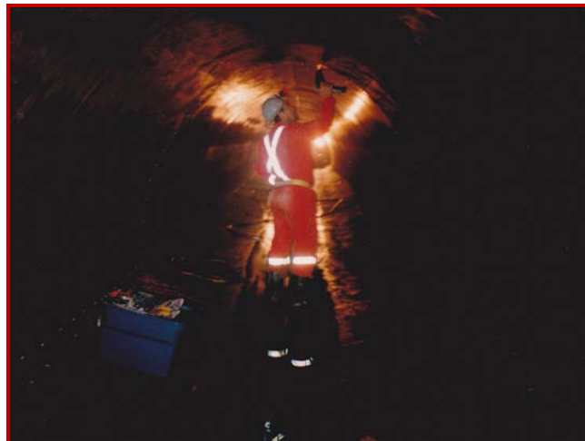
Cracks and construction joints in potable water structures are permanently sealed with FLEXIBLE RESIN.
