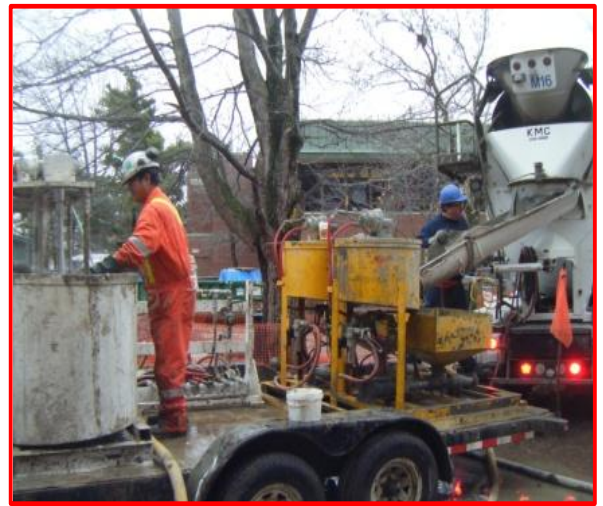
Excavation contractors rely on Multiurethanes' products, such as CELBEX 653, to stabilize weak ground conditions.
