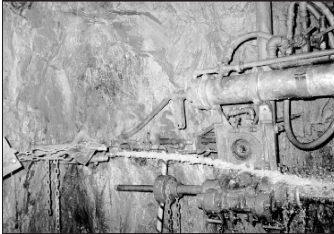
Underground drill hole showing the result of intersecting water-bearing fractures at a depth of 500 feet below surface; water pressure testing established that rock fissures were very narrow, thus justifying the use of microfine cement grout
