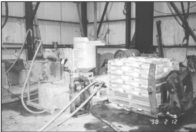
This mine shaft grouting operation utilized a colloidal grout mixer for preparing high-quality ordinary Portland and microfine cement grouts, in conjunction with a grout agitator tank and a low-pressure, high-volume diaphragm pump suited for site conditions; actual grouting pressures within the shaft were higher than pump pressures due to the effect of gravity.
