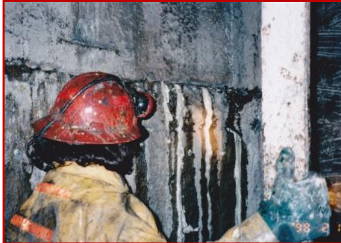
MME UNIVERSAL RESIN is used to stop water inflows through leaking concrete construction joints in an underground mine shaft.
