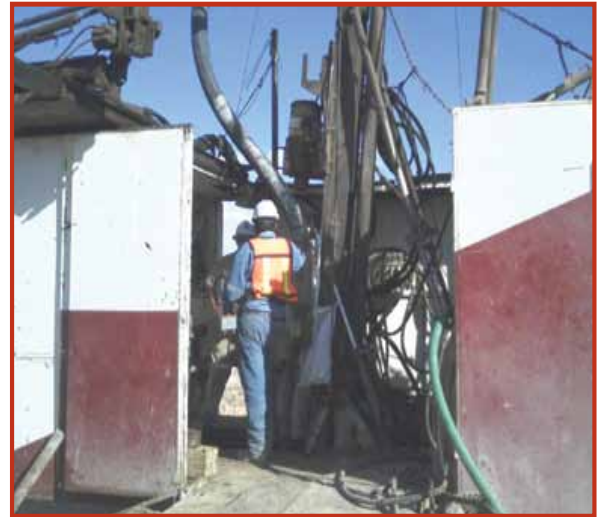
Excellon Resources, Platosa Mine, Mexico Deep hole drilling and high-volume cement grouting operations were used to seal water-bearing rock formations and successfully recover a flooded underground silver mine.
