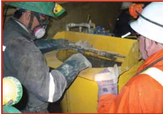
Pan American Silver, Huaron Project, Peru Cement grouts were used to reduce high volume water inflows through fractured and water-bearing ground conditions prior to shaft construction using conventional sinking methods.
