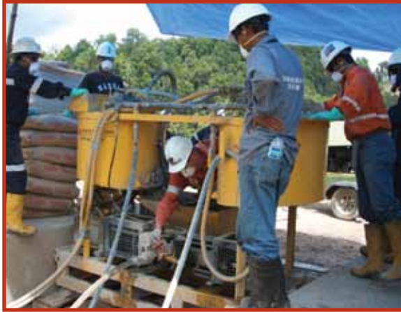
Newcrest Mining, Kencana K2 Project, Indonesia Microfine cement grouts were used to improve ground conditions through fractured and water-bearing ground conditions prior to ventilation shaft construction using raise bore methods.
