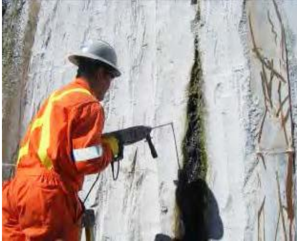
Chemical Grouting (Niagara Falls, ON) Supported an extensive rehabilitation project for a leaking rock shaft at a hydroelectric dam.
