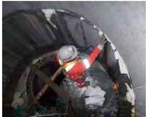
Water Cut-Off (Mississauga, ON) Worked on-site to seal active infiltrations through pre-cast manhole segments.
