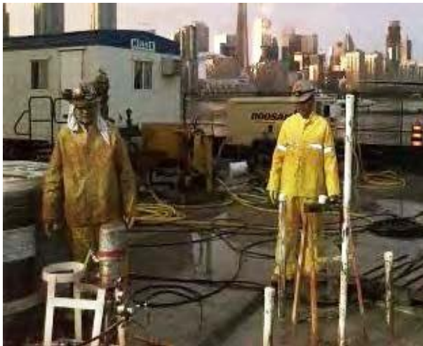
Soil Stabilization (Toronto, ON) Applied a grouting solution involving sodium silicate, delivered through sleeve pipes, after surface voids formed during a directional drilling project beneath an airport construction jobsite.
