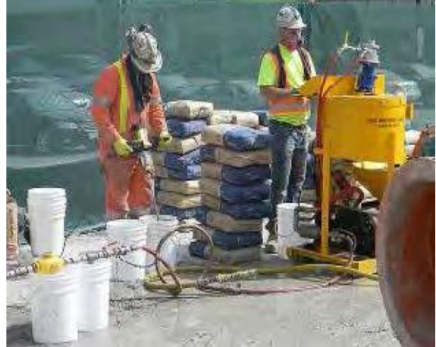
Cement Grouting (Toronto, ON) Performed microfine cement grouting and sodium silicate grouting for soil stabilization in cross-passage tunnels along the road in a light-rail transit (LRT) line construction project.
