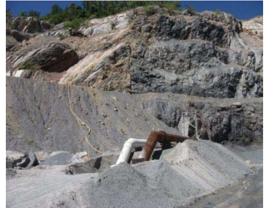
Several full-scale mockups were constructed to observe various aspects of the grouting operation
